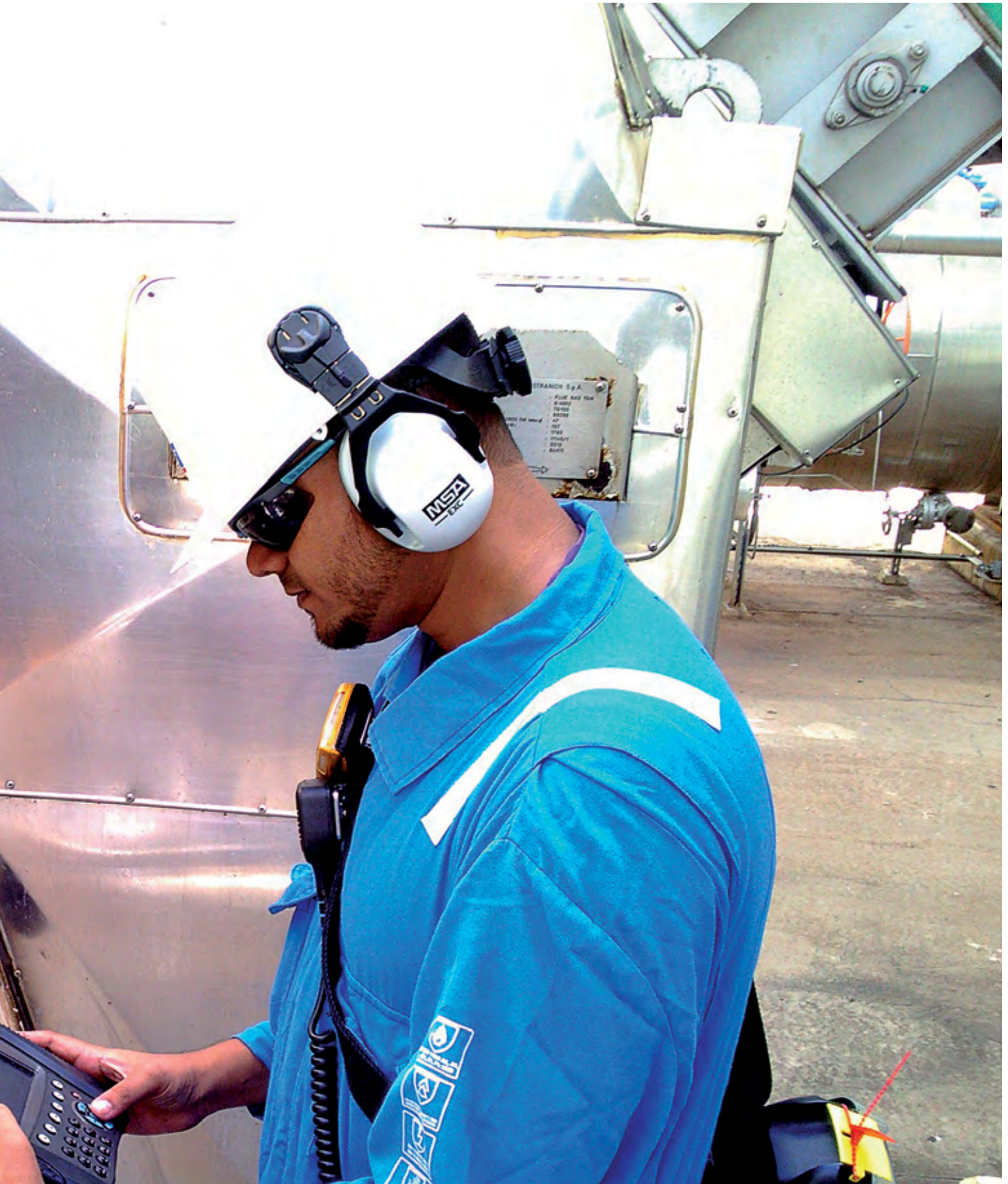
■ ■ An operator doing maintenance on a pump in a unit of the Staatsolie refinery.
