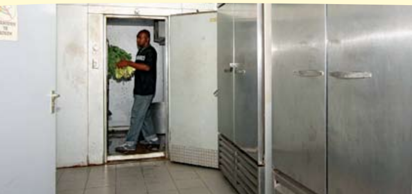
Improved food safety for the 350 elderly residents of Huize Ashiana, through renovation of the kitchen.
