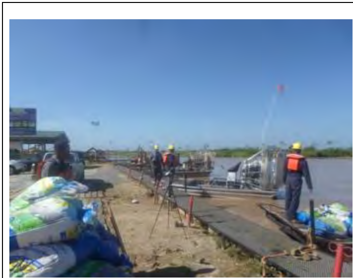
Location NU01: At the quay near the transfer station (90 m from the pump station). Airboats/boats are starting and arriving on spot. Material is being loaded on the airboats.
