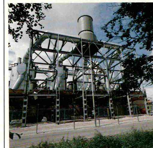
Central steam installation. (Schoonebeek steam injection area)
