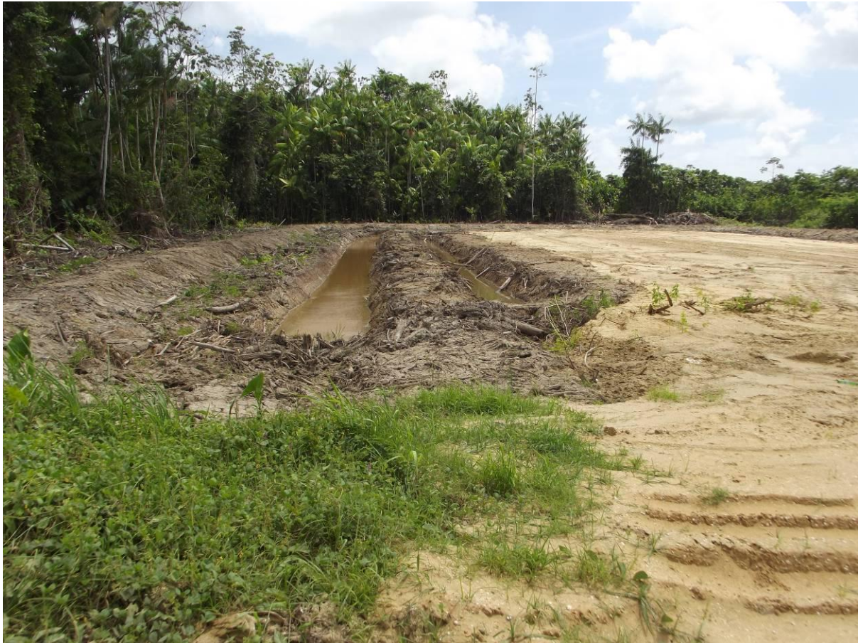
Figure 8: Drill site, with from left to right, the outer dam, the perimeter ditch, the mud pit, the inner dam and the sandy drill platform.
