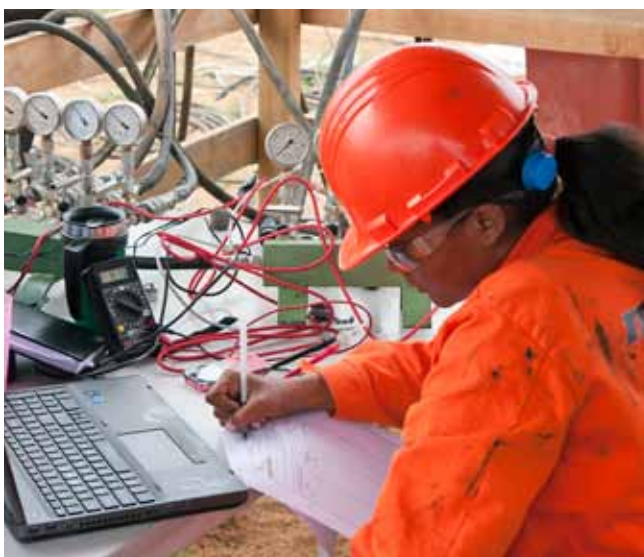
While a pile driver knocks a concrete pile in the ground, a site worker measures the vibrations.
