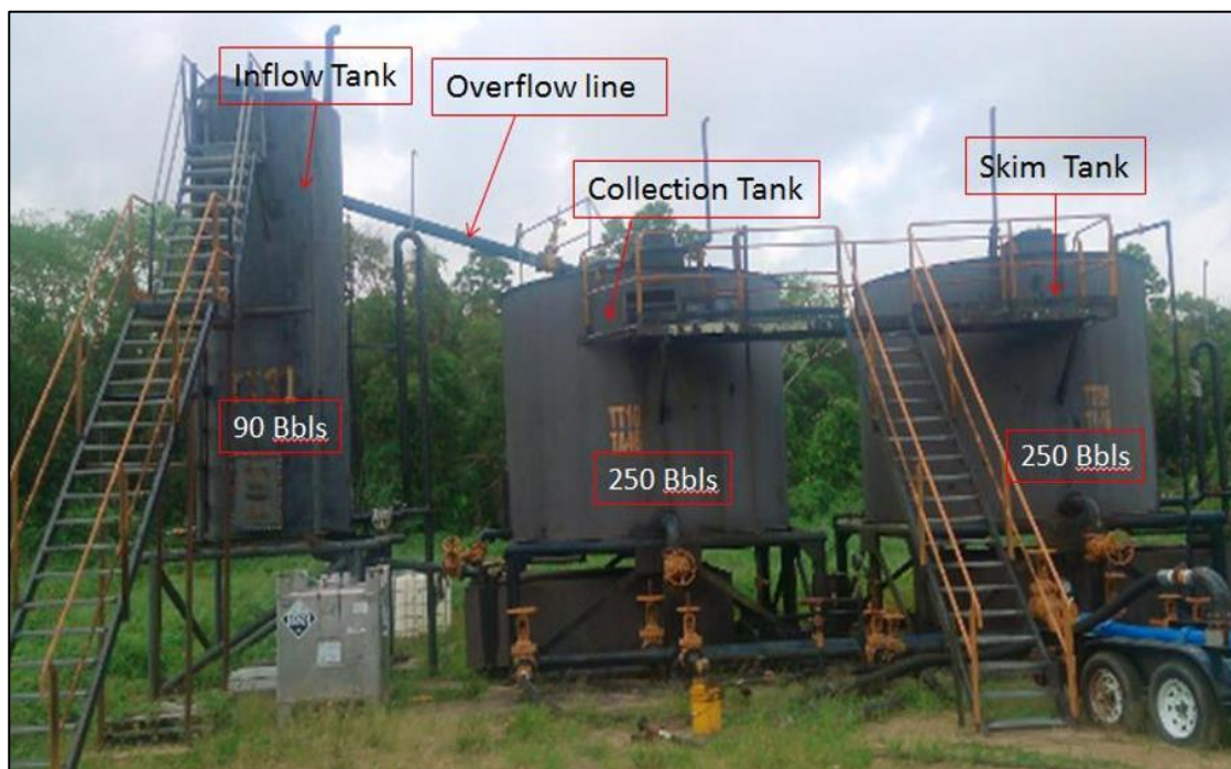
Figure 3-10: Produced water separation facility at TA46 test station 10/11
